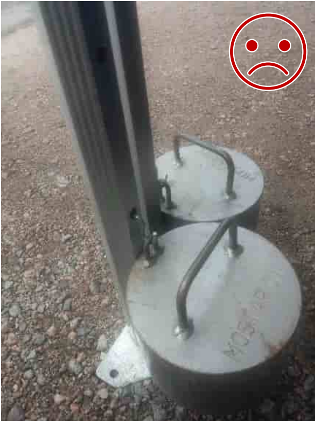
Figure 9 WRONG. The steel hook does not lock into the structure, and the steel will cut the aluminium as lift shakes the tent.
