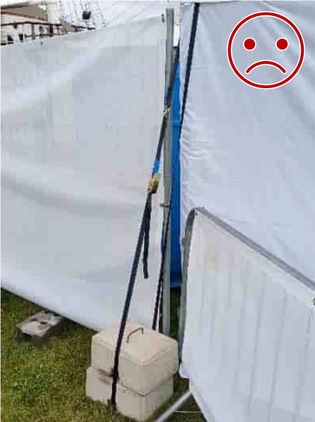
Figure 11 WRONG . The weights are not locked to the strap or to each other. The stack will fall, and the strap will not hold as the structure shifts.
