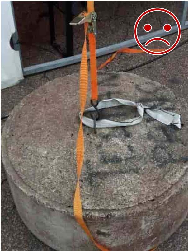
Figure 7 WRONG. The S-hook is not lockable. The hook will come loose as the structure shifts.
