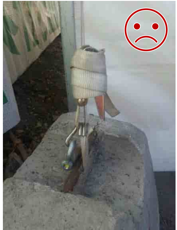
Figure 6 WRONG. The hook is not locked, should be locked with a shackle to the fixing point.
